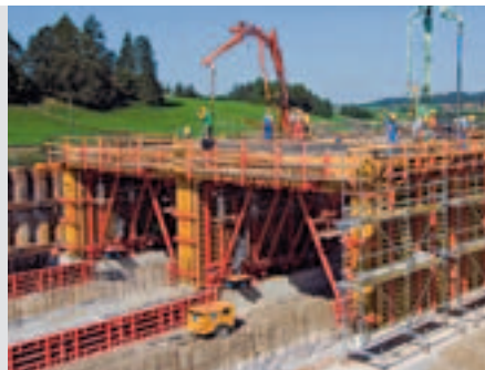
Final assembly on the jobsite Final assembly of large formwork projects is carried out on-site.
