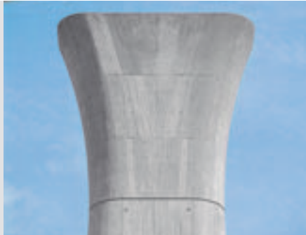
Exact and with the required board structure – one of altogether 16 pier heads after completion.
