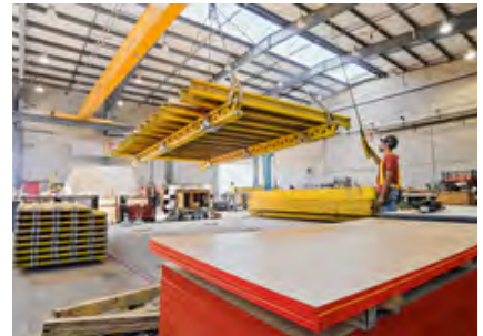
The pre-assembly at the PERI factory is also an option available space or timeconstraints do not allow the assembly on site.
